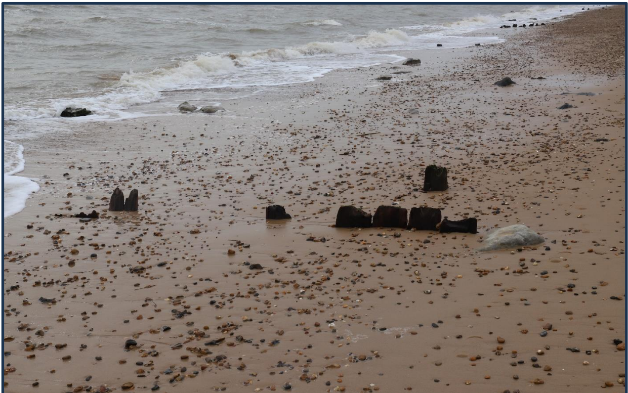
Photo 2: View of remainder of groyne on the foreshore, looking south
